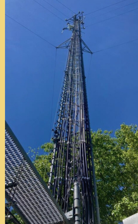
Radio tower in Lincoln County.
